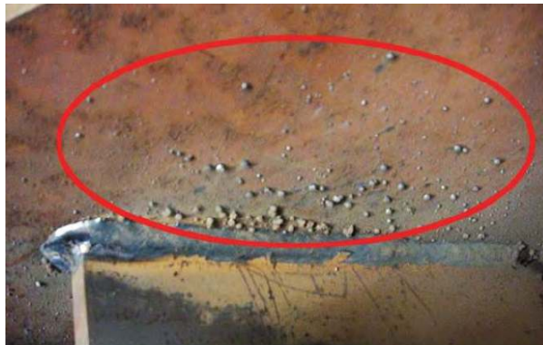
Gambar 8.21 Cacat spatter . Sumber: American Welding Society 2015
