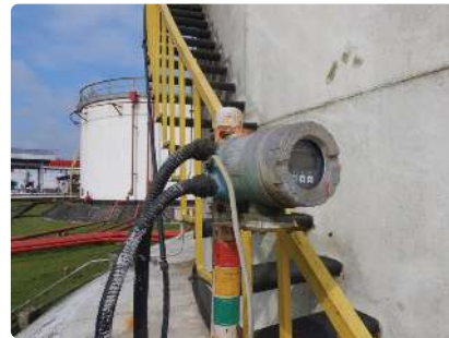
Gambar 8.9 Automatic Tank Gauging (ATG)
