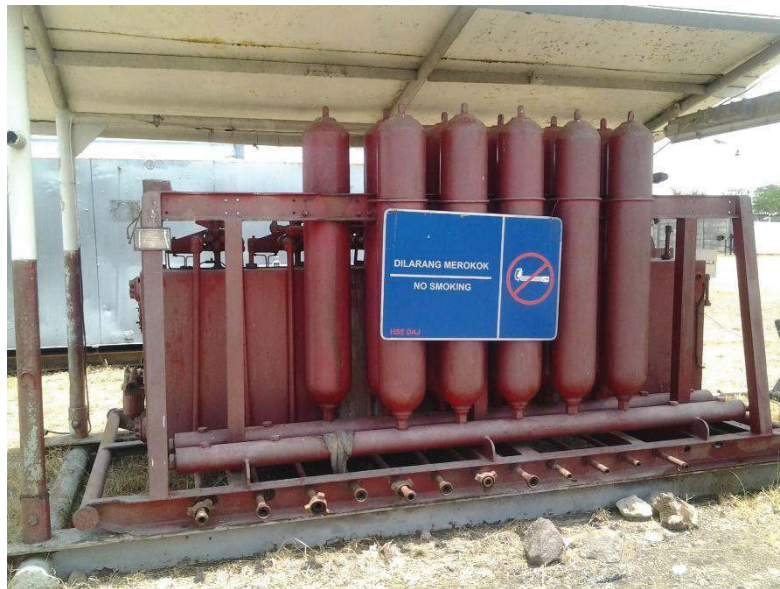
Gambar 6.28 Accumulator Sumber: Yudanto (2014)
