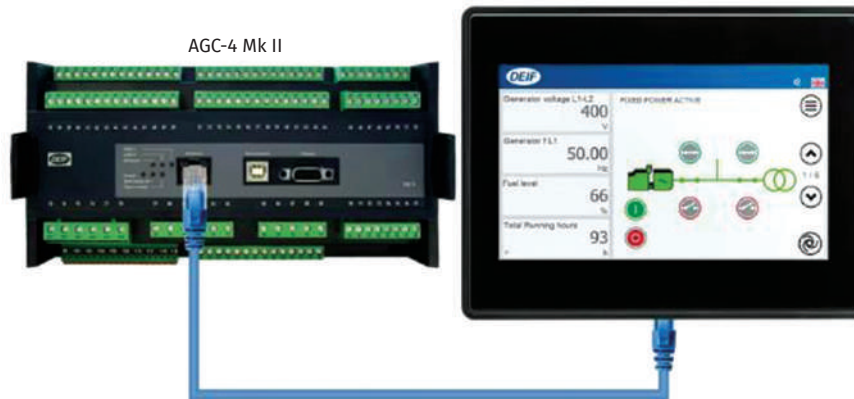
Gambar 4.18 Generator Synchronization Controller Sumber: DEIF (2024)
