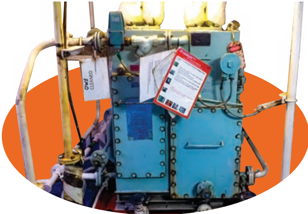
Gambar 7.5 Oil Water Separator
