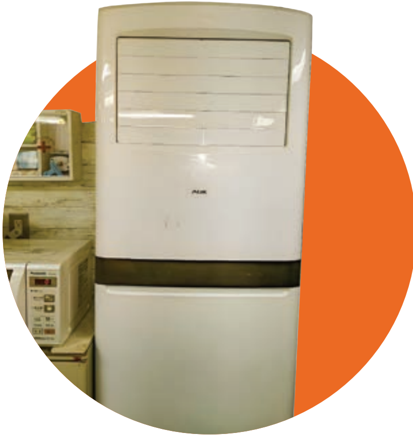
Gambar 4.17 Sistem pendingin ruangan di Engine Control Room (ECR) Sumber: Fino Waspodo (2024)
